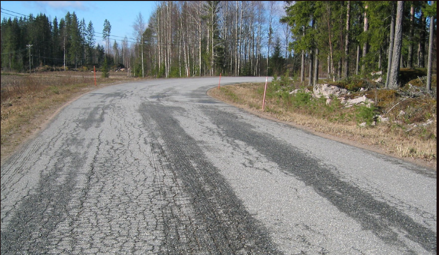
Rutting in evidence: It occurs because the layer of pavement below the seal is compressed, resulting in a set of continuous ruts occurring in the lane mirroring the track width of the tyres of trucks and trailers.
