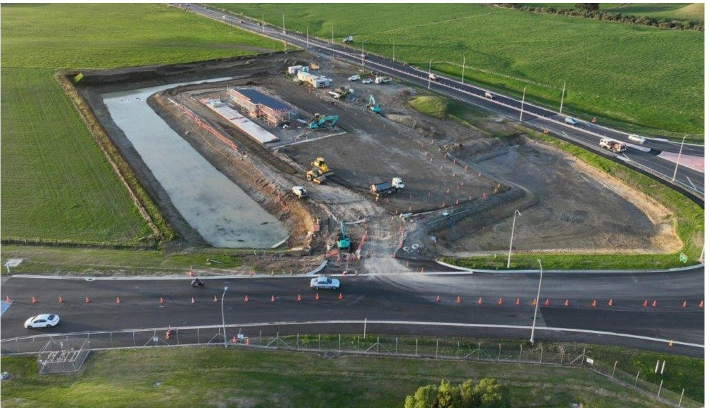
The new Commercial Vehicle Safety Centre (CVSC) under construction at Ohakea will be one of 12 such centres planned nationwide.
